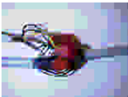
Figure 3: Wiring effort to connect one double valve with sensor to the matrix cables
